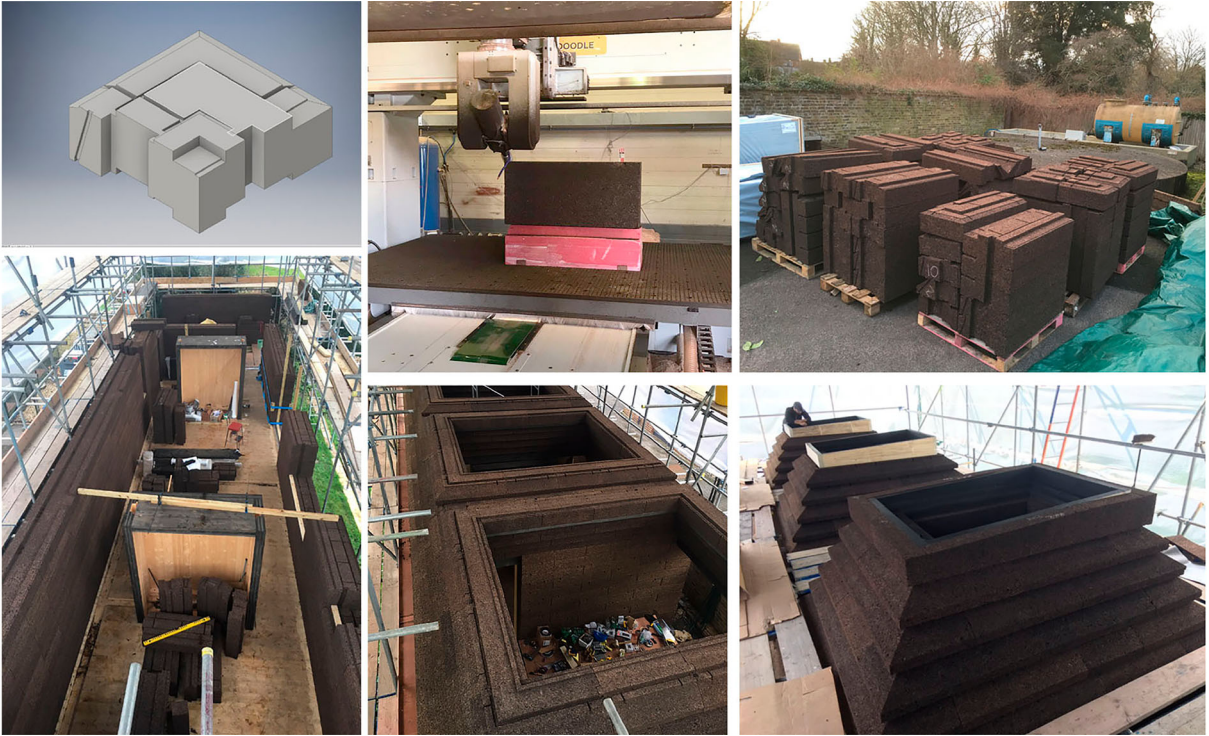
Figure 11. (top, from left to right) Model of corner wall block profiled to accept door frame, CNC milling a block, wall blocks on site ready for assembly; (bottom) assembling the walls and roof, © Matthew Barnett Howland
