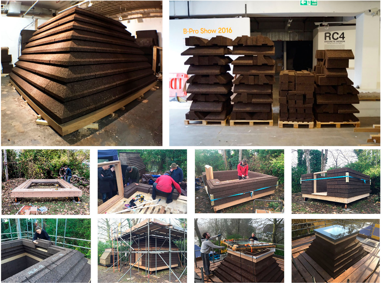
Figure 8. (top) Cabin roof assembled to check fit at The Bartlett then disassembled for transport to site; (bottom) Cabin assembly on site, © Oliver Wilton and Matthew Barnett Howland
